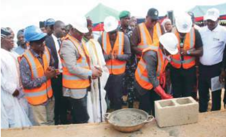
Governor Lalong laying the foundation stone being witnessed by Alhaji Suleiman Abubakar of Imani Groups, Aburime Pollard, MD/CEO, Drallop Services and others
