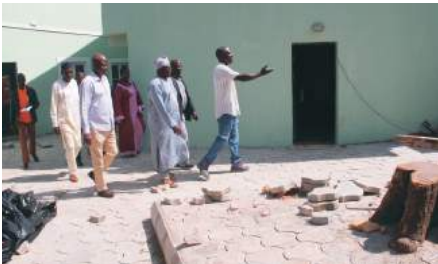
Engineer handling the remodeling of the NUJ Secretariat, Engr. Yarima Balami (right) taking the team round the project site
