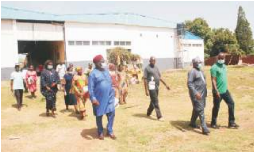
Acting General Manager, Mr. Paul Jatau (right) conducting the Commissioner, Hon. Dan Manjang and team round the ongoing renovation of PPC
