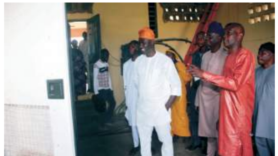
Commissioner at the Generator room of PPC listening to the Director of Technical Service, Elder Dapas Elkana
