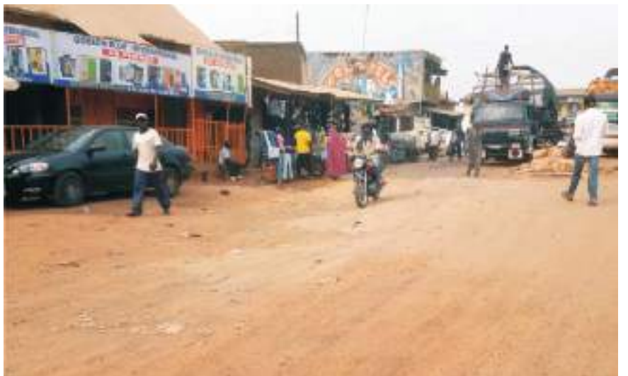
This road from Bauchi Rd junction to Bayan Banki washed out completely
