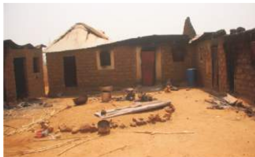
Burnt house at Kwashaslalek, Mangu LGA
