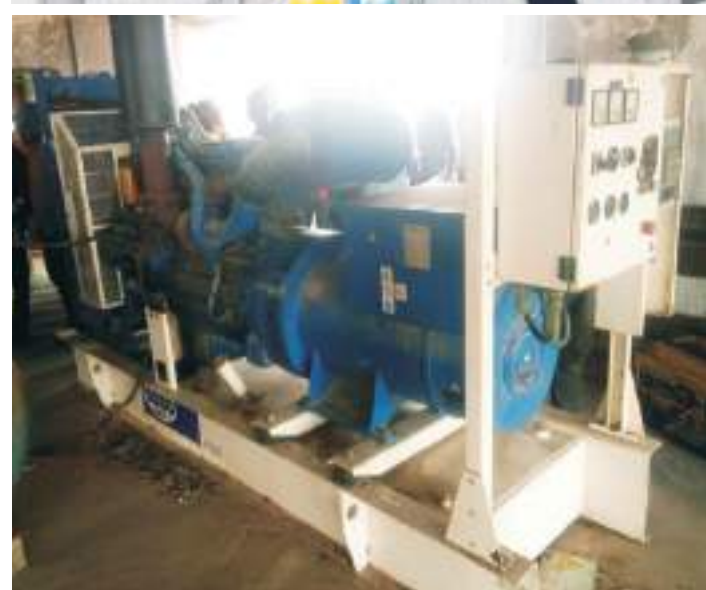
Bokkos treatment plant
