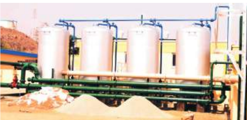
Work on the water treatment plant being carried out by the ministry of Water Resources and Energy at Langtang North LGA
