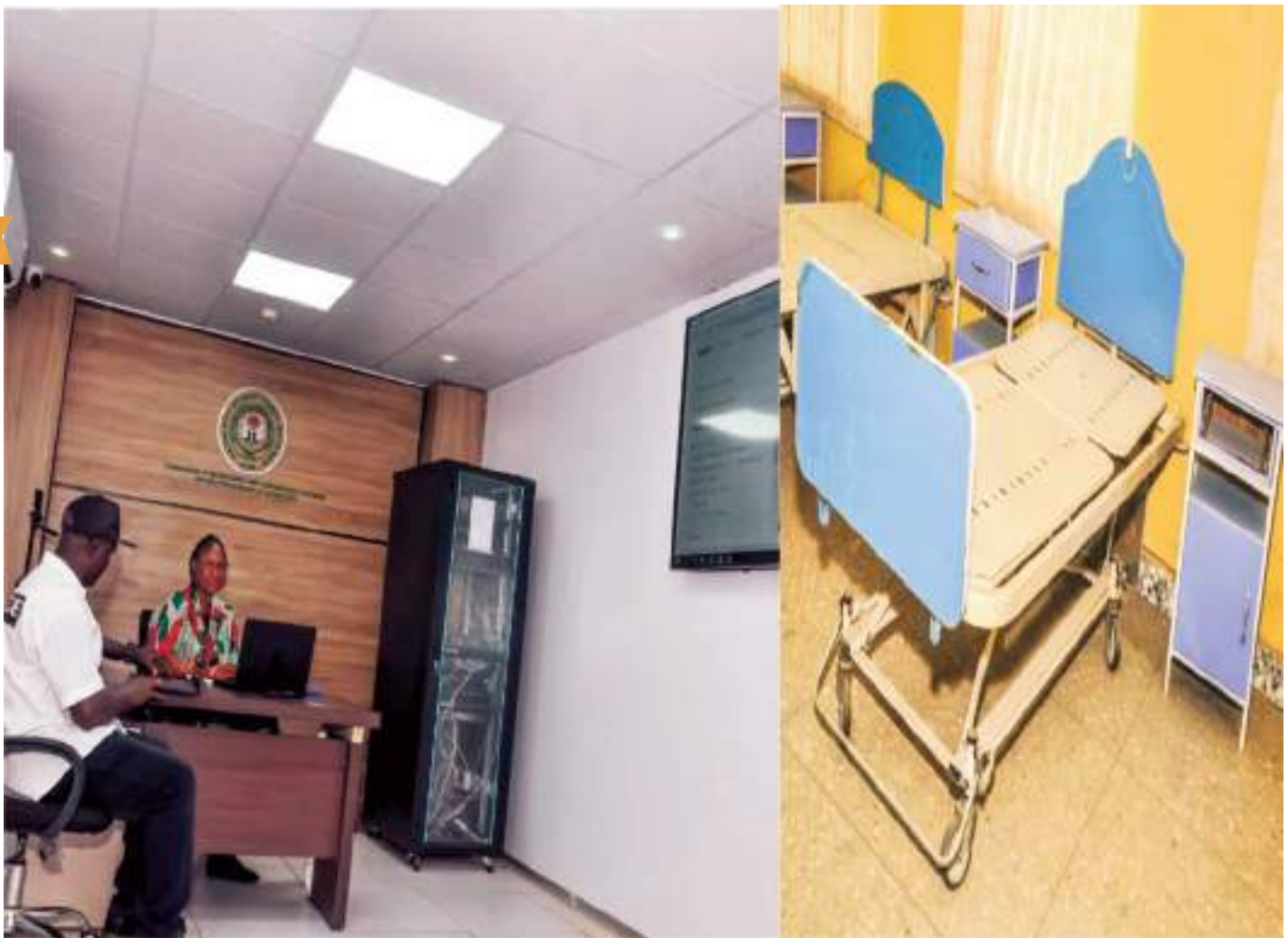
PSSH Server Room (EMR)
